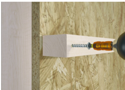
Mounting of installation level
